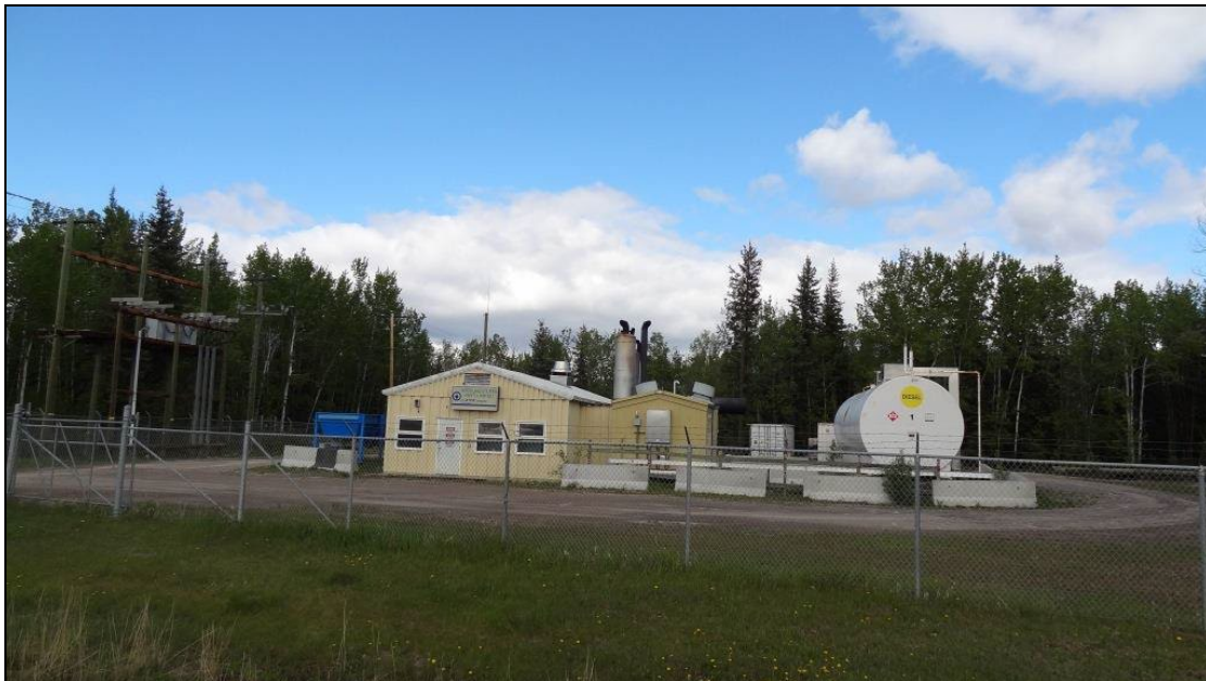
Northland Utilities Diesel Power Generation, Fort Providence
