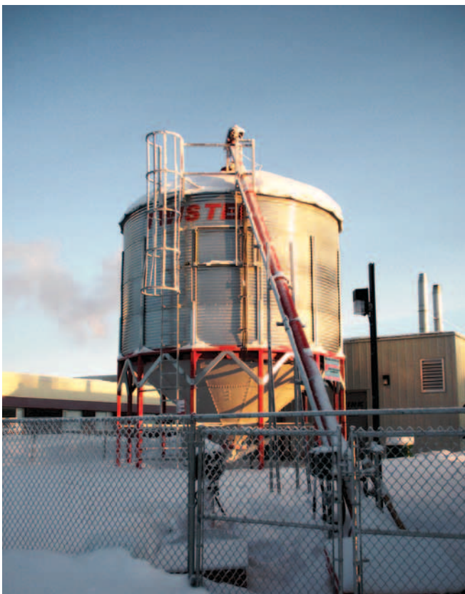
Wood pellet boiler installation at Chief Jimmy Bruneau School in Behchoko – Photo Credit: PWS/GNWT
