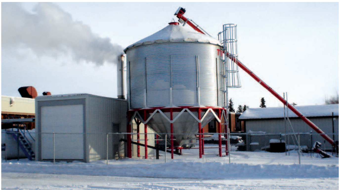
Pellet boiler installation at Chief Jimmy Bruneau School in Behchoko - Photo Credit: PWS/GNWT
