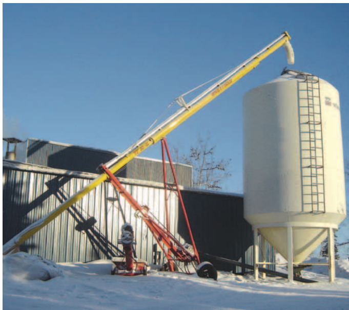
Pellet boiler installation at Sir John Franklin High School, Yellowknife - Photo Credit: Arctic Energy Alliance
