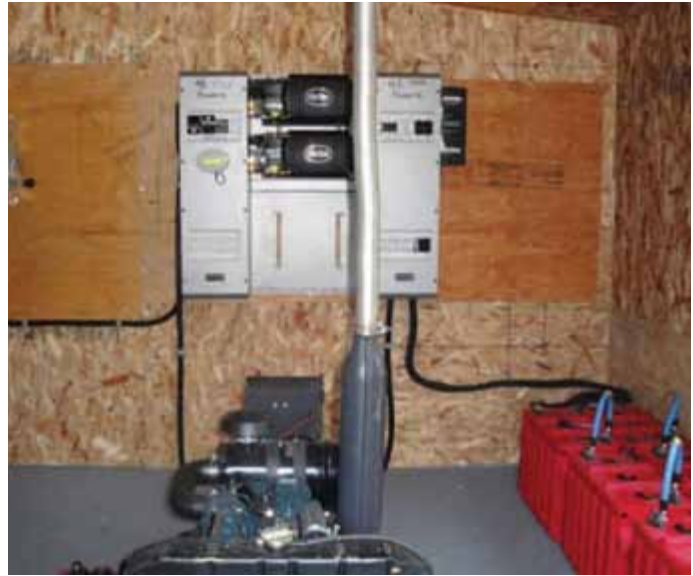
Enodah Wilderness Adventures, Off-grid Solar Battery Charging System, Installed 2010 – Photo Credit: Ragnar Wesstrom
