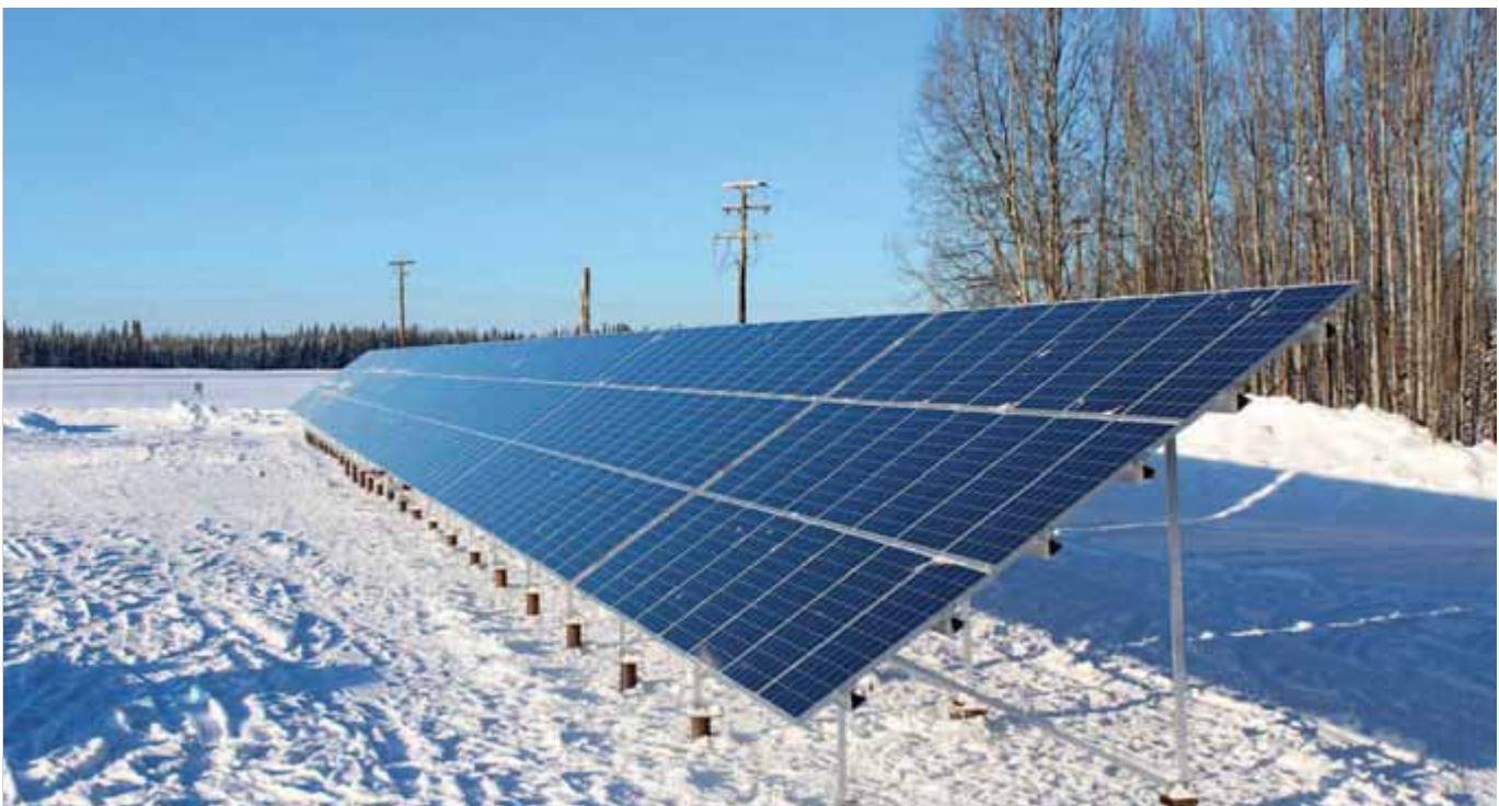
Fort Simpson, NTPC 60 kW Array. Installed 2011 (2) – Photo Credit: NTPC
