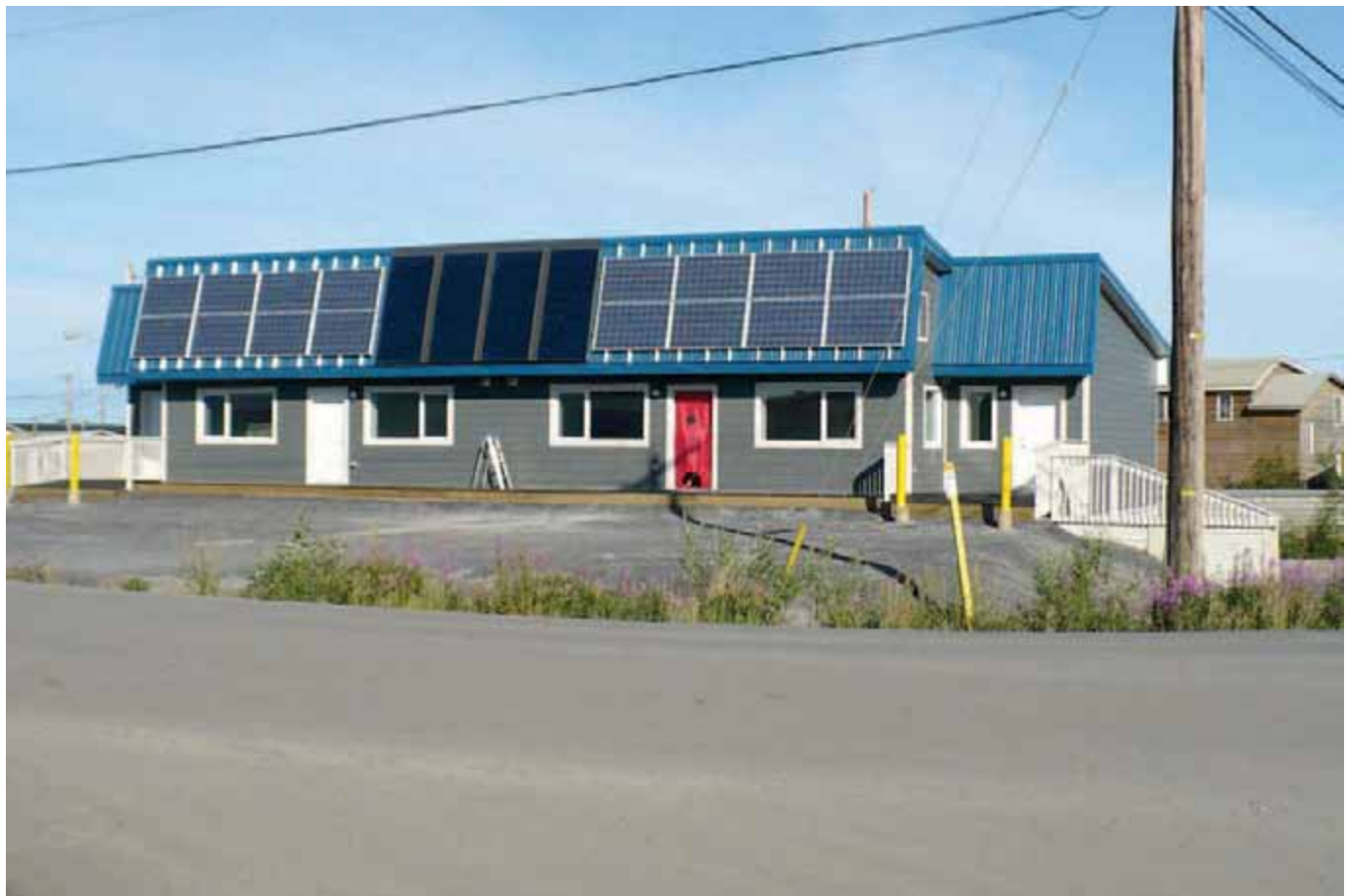
Northern Sustainable Housing Project, Inuvik, Solar PV and Solar Hot Water, Installed 2012 – Photo Credit: Wade Carpenter/GNWT
