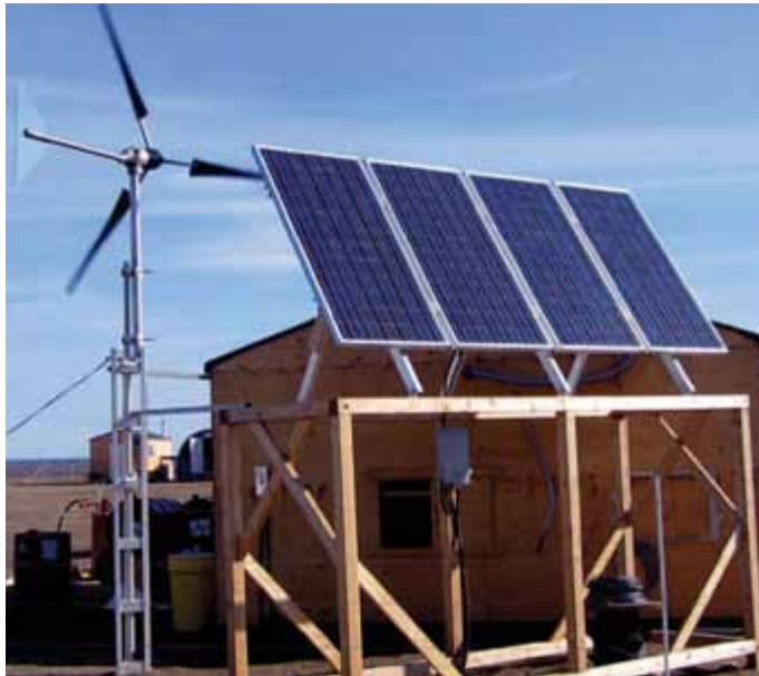
Rio Tinto Exploration Camp, Banks Island. Off-grid Battery Charging System. Installed 2011 – Photo Credit: Paul Jones
