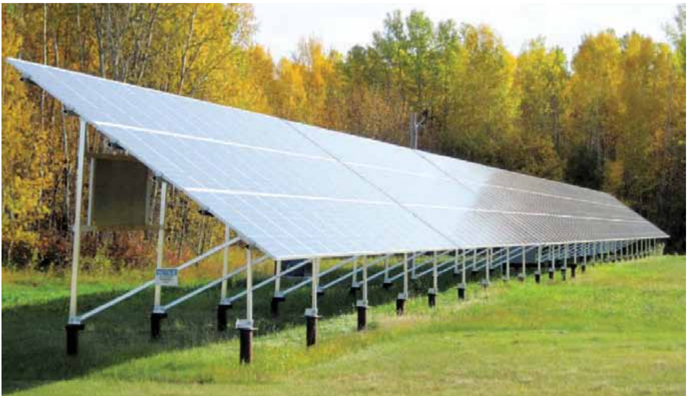
Fort Simpson, NTPC 60 kW Array, Installed 2011 - Photo Credit: Melanie Burgess
