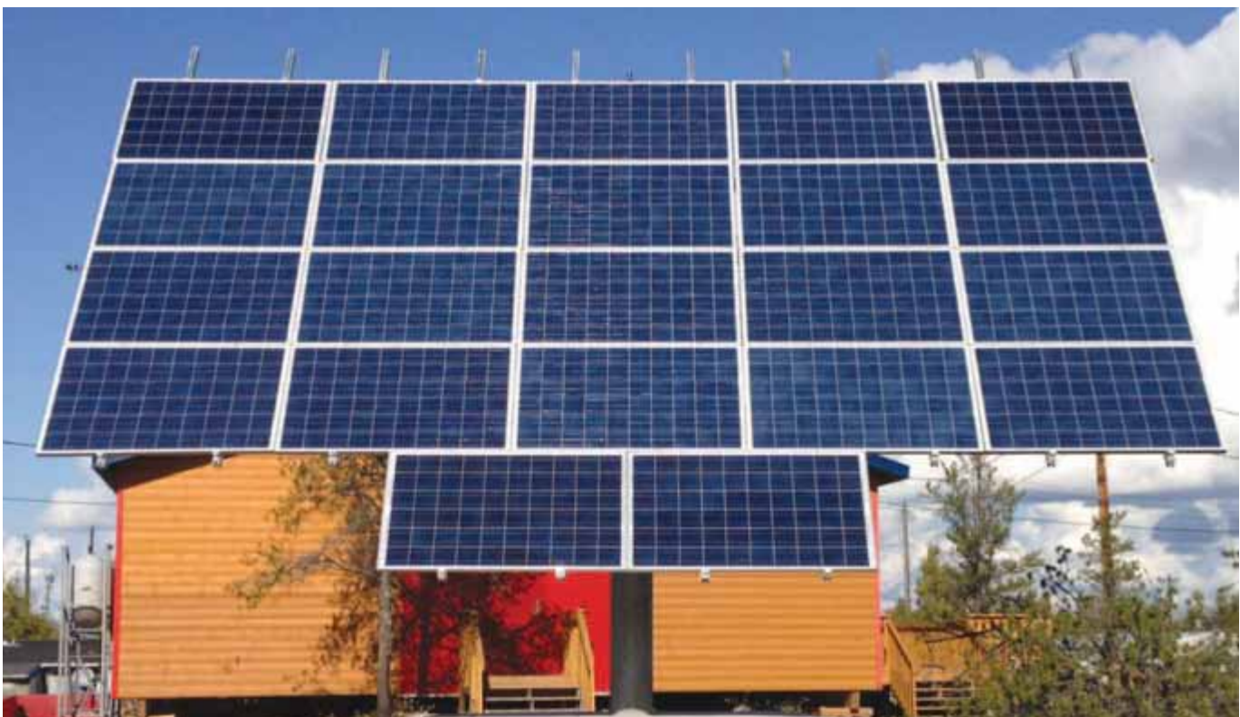
Edzo Youth Centre, 5 kW Dual Axis Tracker, Installed 2012 – Photo Credit: Matthew Brost
