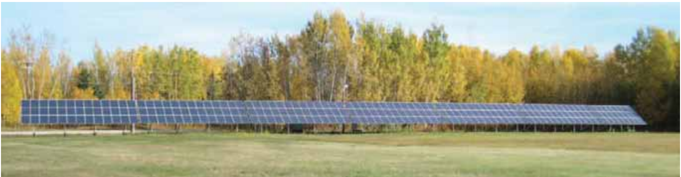
Fort Simpson, NTPC 60 kW Array. Installed 2011 – Photo Credit: Melanie Burgess
