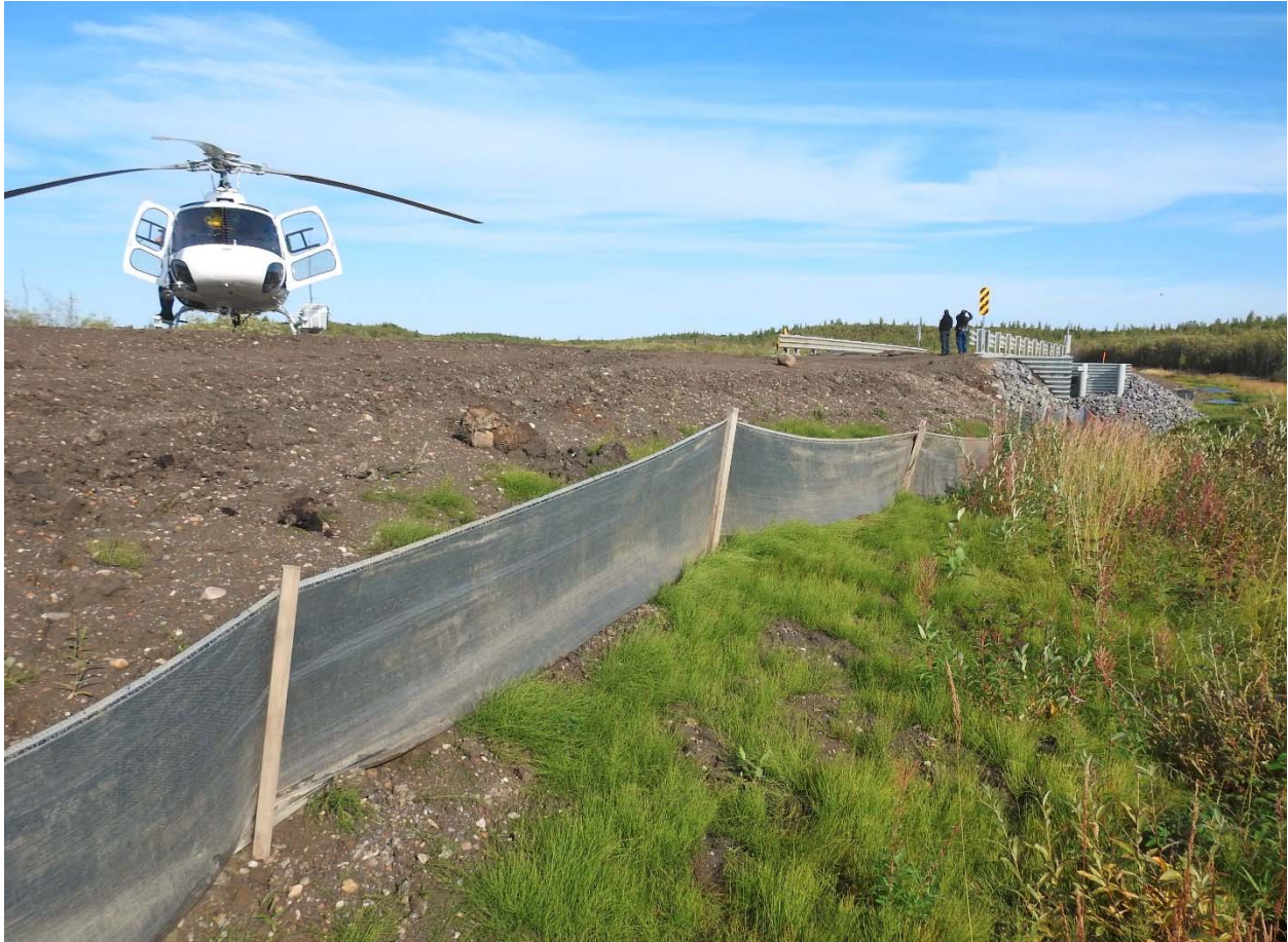
Figure 12. Survey site at bridge crossing along the Inuvik to Tuktoyaktuk Highway route.
