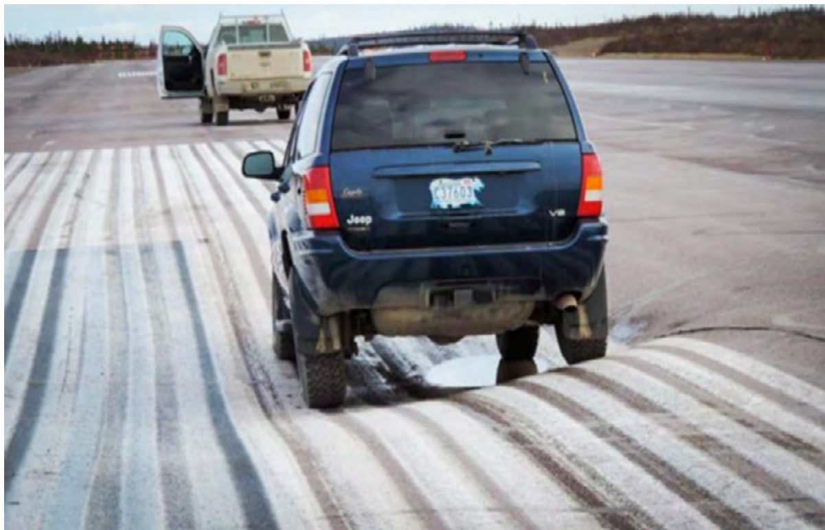
Figure 6. Dip in the Inuvik Airport runway caused by permafrost thaw. Source GNWT.
