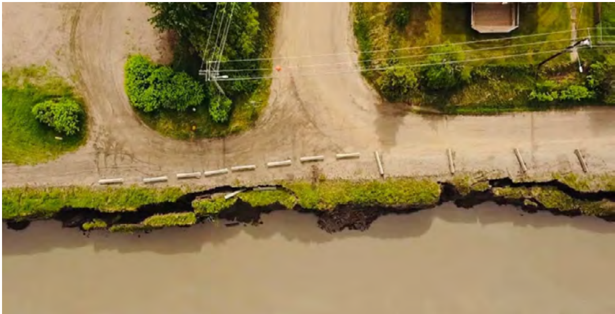
Figure 8: Riverbank erosion in Fort Simpson. Photo courtesy of Brandon Buggins.
