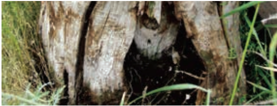
Wooden pilings rot over time in warm, moist conditions
