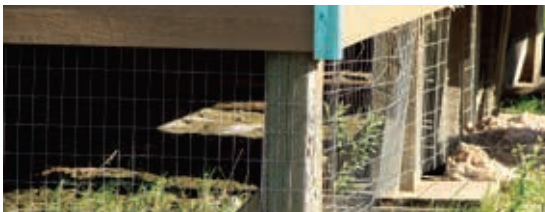
Wire mesh allows airflow but keeps foundation clear
