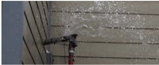
Overflow from your water tank builds up Photo credit: NWT Housing Corporation
