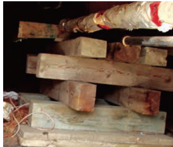
Permafrost degradation affecting foundations
