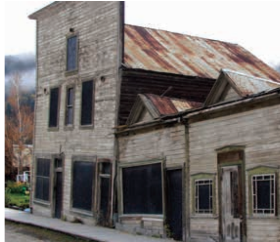
A structure with foundation issues due to permafrost
