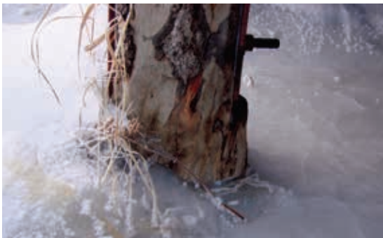
Ice and water causes rotting of piles
