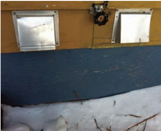
Dryer vents should not be vented into crawl spaces
