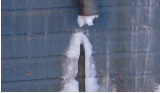
Frozen overflow from a water tank Photo credit: NWT Housing Corporation
