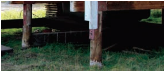
Rotten pilings put your foundation at risk
